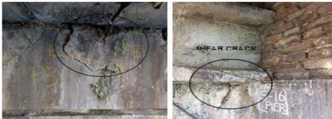
CRACKS ON PIER BEARINGS
